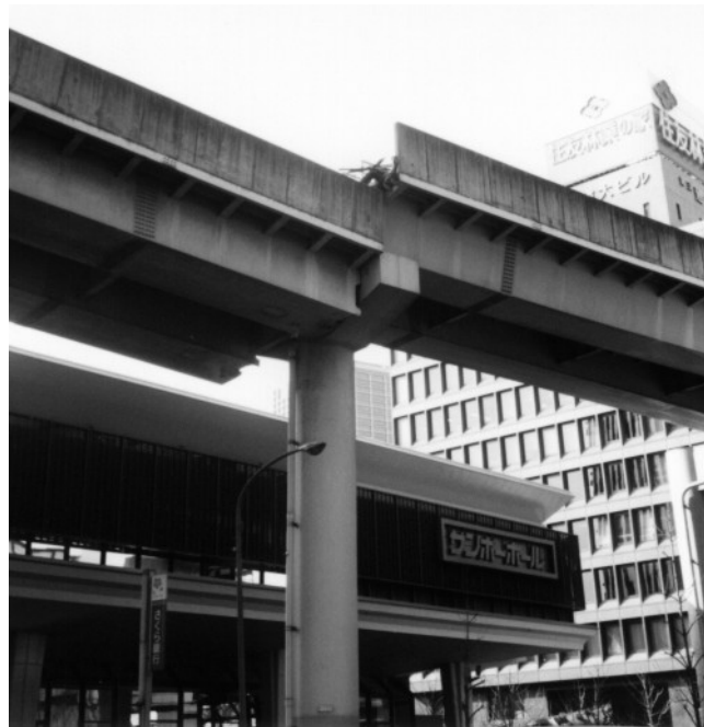
Figure 1: Bridge with insufficient seat length (1995 Kobe earthquake)
