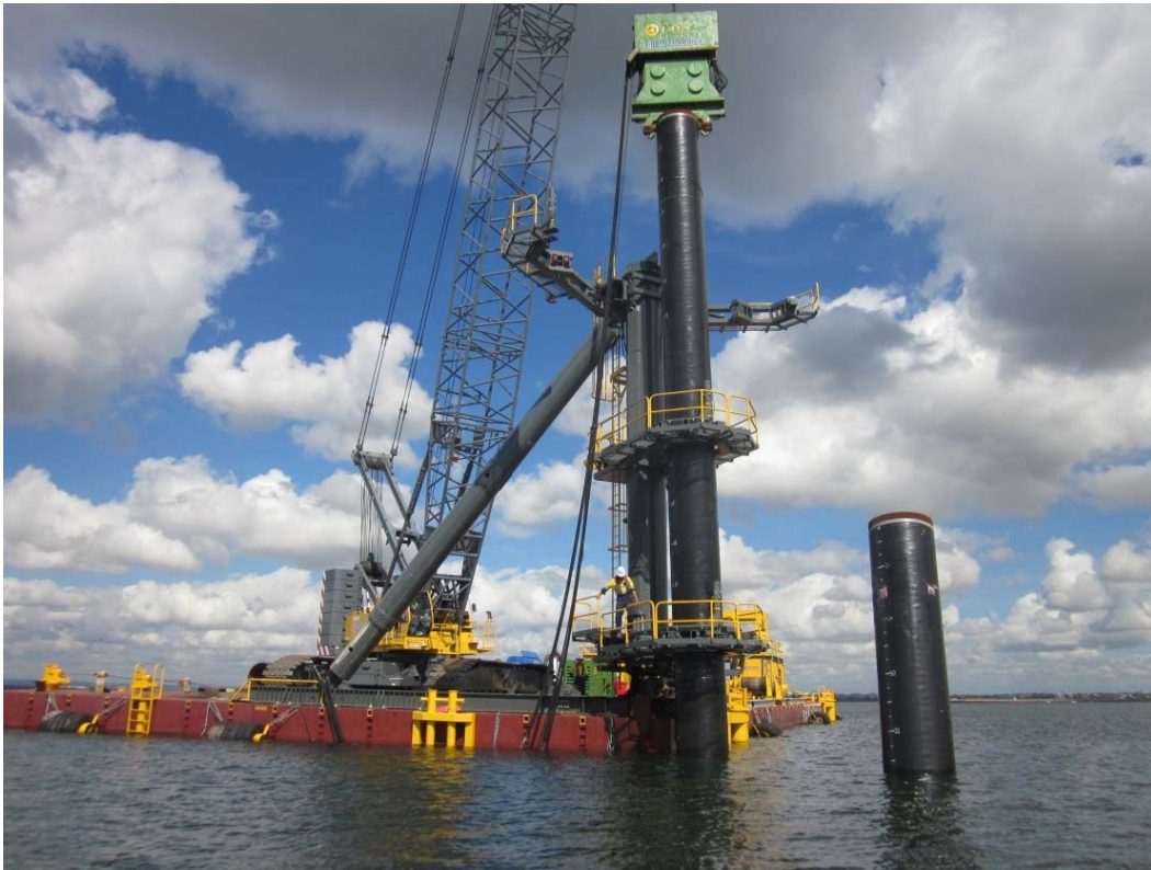
Figure 4. Poseidon flexi-float barge and 250 tonne crane, with pile in the leader using the 14 tonne ICE vibrating hammer to drive a raked pile.
