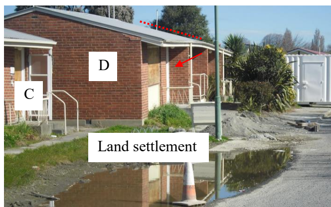
Figure 5 – Building D differential settlement (view roof line). Building ‘broken’ around dotted line.
