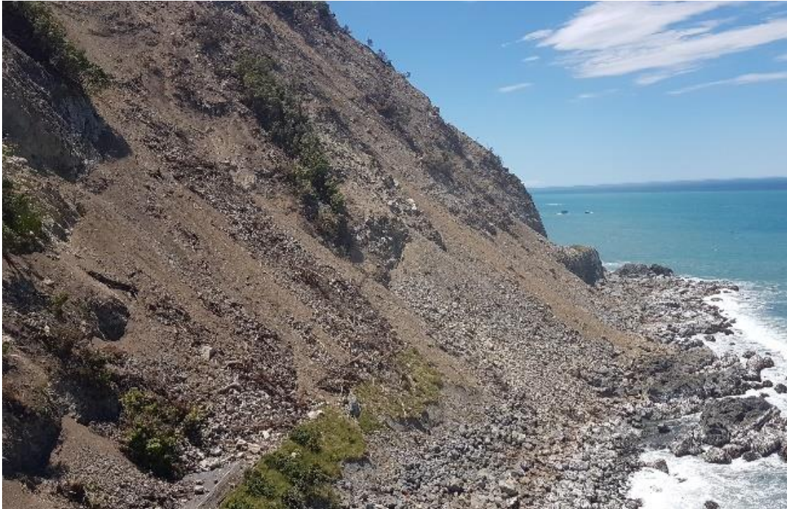
Figure 1: Landsliding on State Highway 1 from 2016 M7.8 Kaikoura Earthquake
