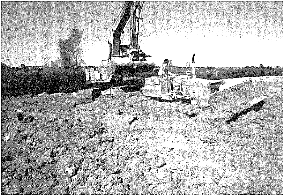
Figure 4. Swamp Track Dozer Stuck in Sensitive Ash Fill
