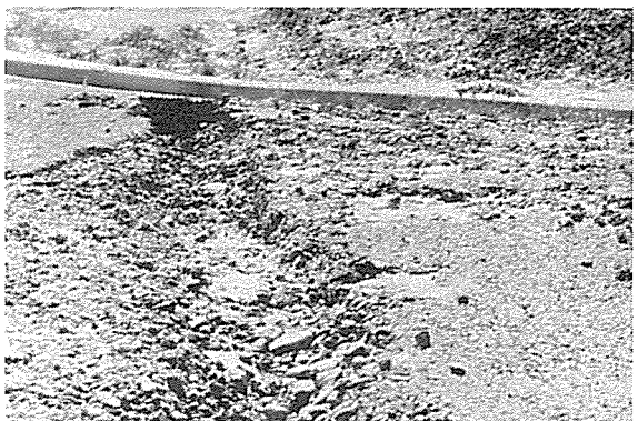
F. SERVICE TRENCH FAILURE AFTER BACKFILLING WITH ERODIBLE LOESS (trench acts as channel-way for water flows)
