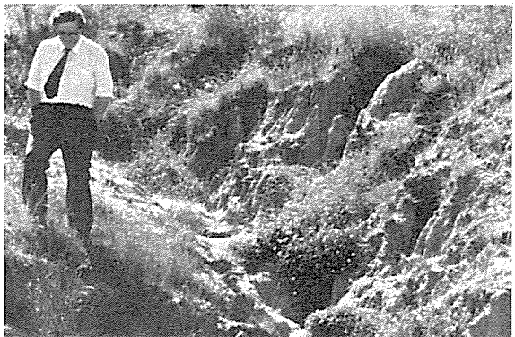
D. SCoured CUT-OFF DRAIN IN ERODIBLE LOESS (trench has gullied down to an erosion-resistant layer)
