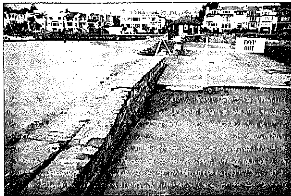
Figure 7 Lateral spreading, settlement, and damage to the seawall at the Marina yacht harbor.
