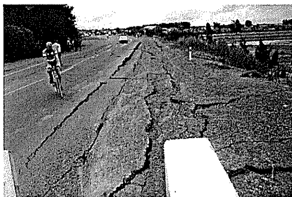
Figure 5 – Damage to the Landing Rd Bridge approach embankment. (Courtesy of H. Chapman)
