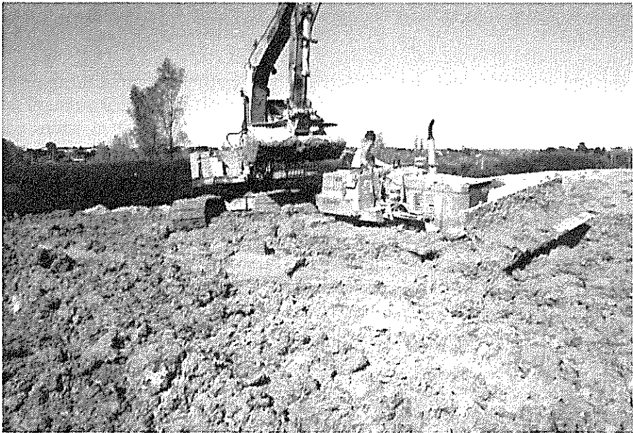
Figure 4. Swamp Track Dozer Stuck in Sensitive Ash Fill
