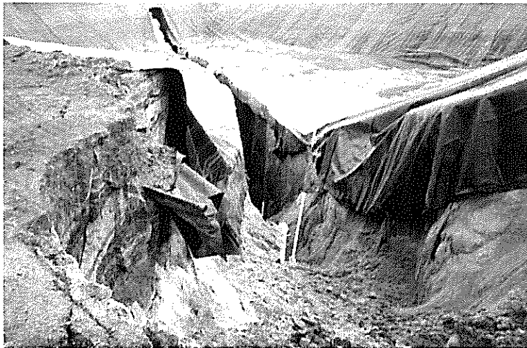
Figure 2. View Along Failed Reservoir from Eastern Corner
