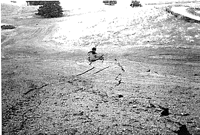
Figure 5. Subsidence Extending Southwest from the Western Corner of the Reservoir. The Gully in which the Water Exited (Figure 6) is Beyond the Far Ridge with Trees
