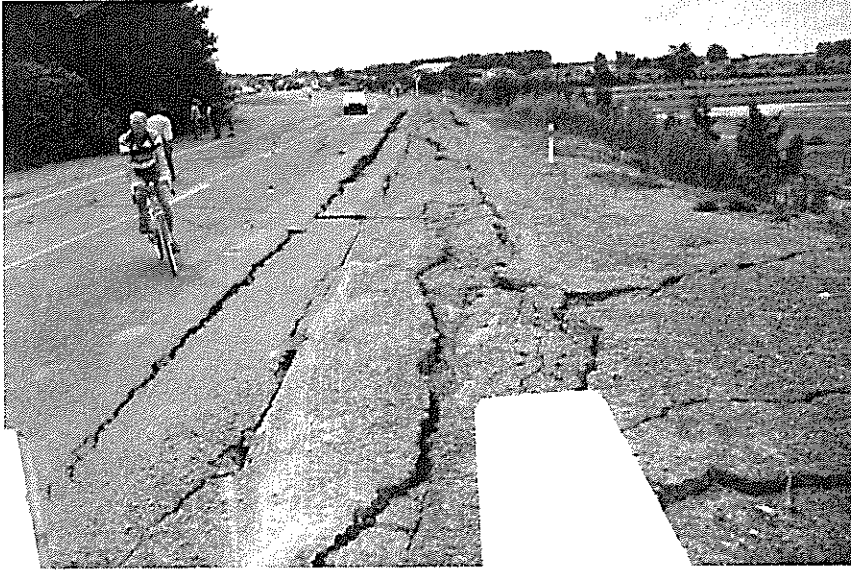
Figure 5. Damage to the Landing Rd Bridge Approach Embankment. (Courtesy of J. Berrill)
