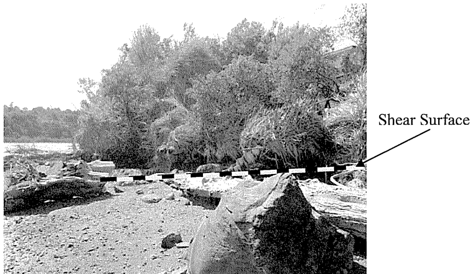
Figure 3: Residual soils sliding over mudstone as seen from shore platform
