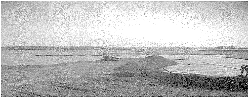
Figure 1: Heap Leach Pad
