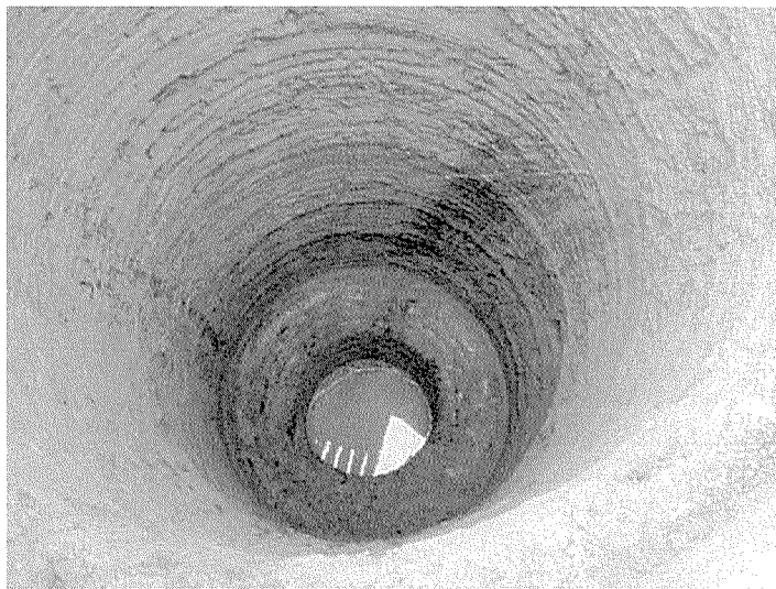
Figure 2: Typical view of a 7m deep, 2.4m diameter pile shaft taken during a site inspection
