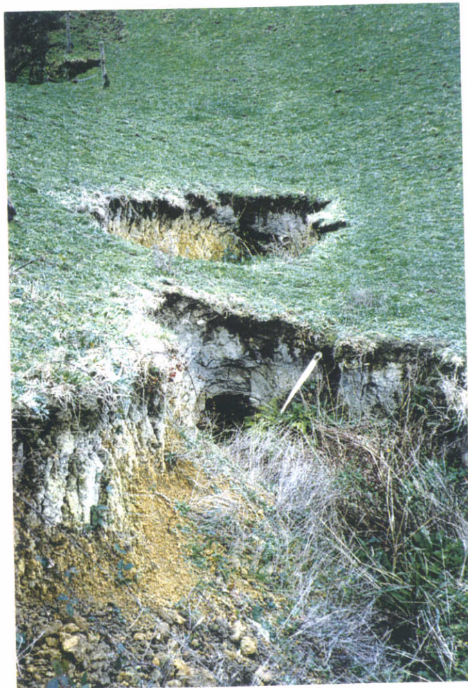
Figure 9 Tunnel gully erosion within soil/rock mass Class A overlying soil/rock mass Class D1.
